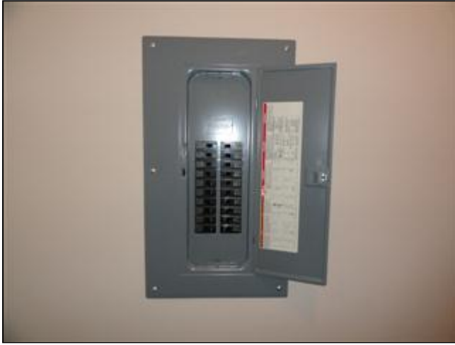
7.6 Picture 3 Sub Panel
