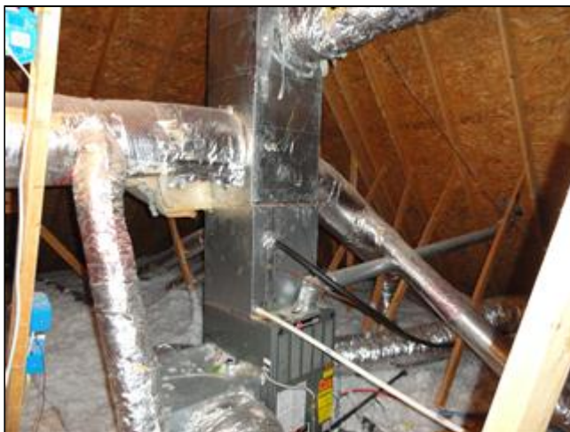
8.11 Picture 2 Furnace in attic
