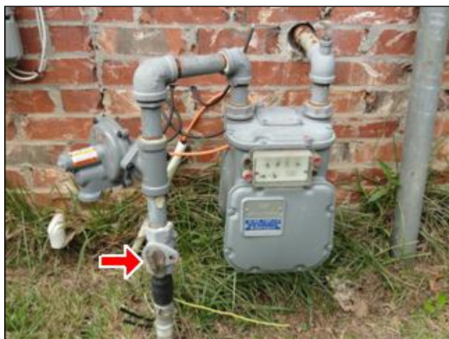
6.5 Picture 1 Main gas shut off
