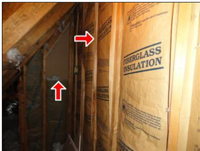
9.0 Picture 2 Vapor Barrier installed backwards and missing
