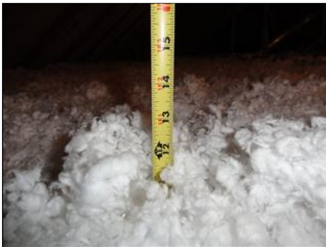
9.0 Picture 1 Blown attic insulation
