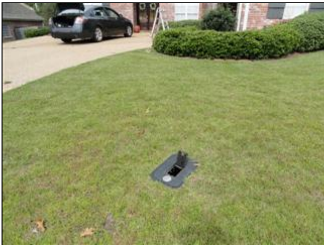
6.3 Picture 1 Main water shut off
