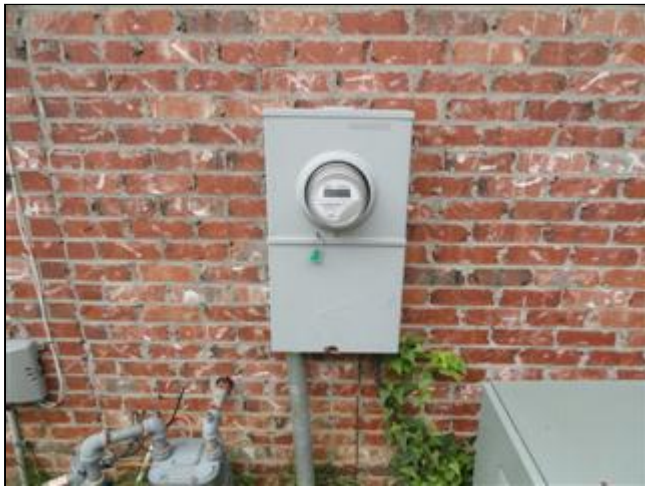
7.6 Picture 1 Main Panel
